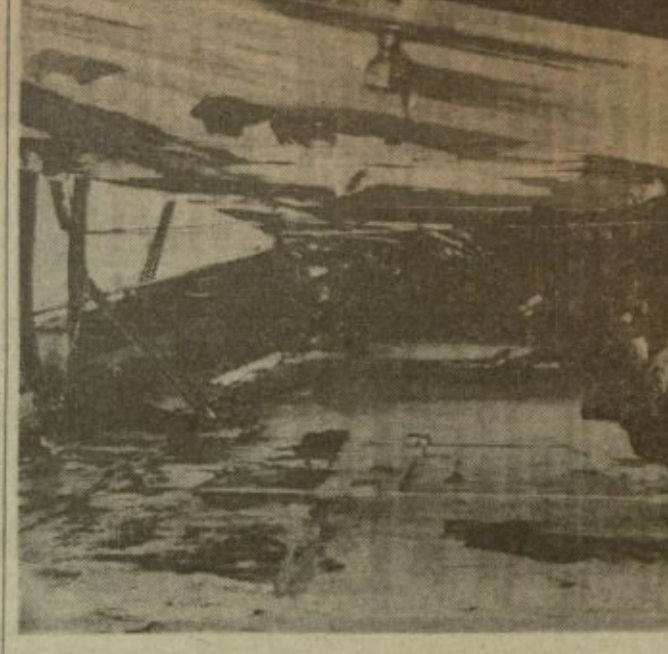
from David A. Morrison, manager of supply house, who hazarded guess that fire was due to short-circuit in conduit of air-conditioning system shown completely charred. —Staff Photos by Sherman S. Skeete
