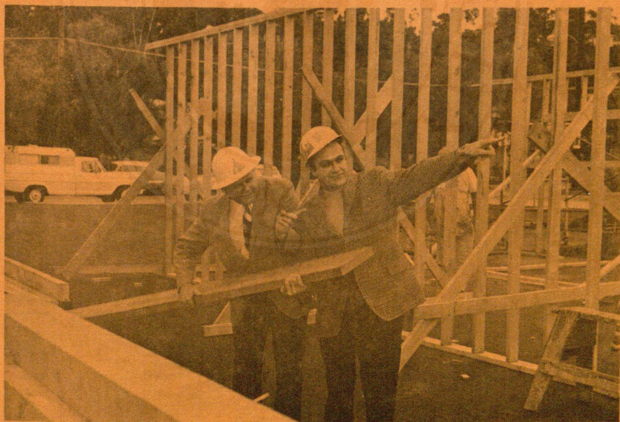
Workers are busy with the renovation of San Diego's "Old Town" in preparation for its opening in May.
